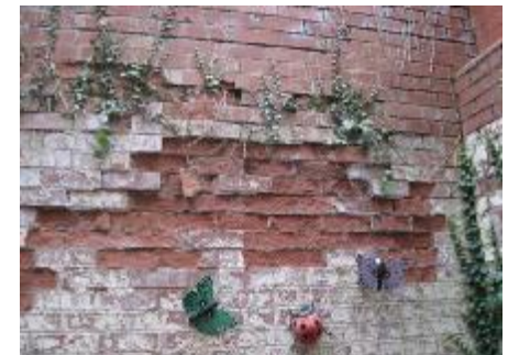
Example of weathered brickwork
