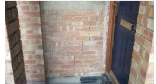
Example of vertical and diagonal cracking
