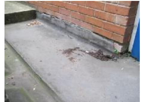
Example of damaged and poor condition asphalt
