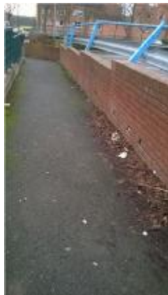
Existing poor condition hard landscaping
