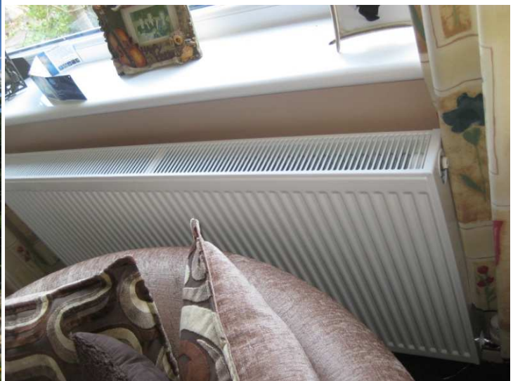
Figure 7: Gas central heating installed
